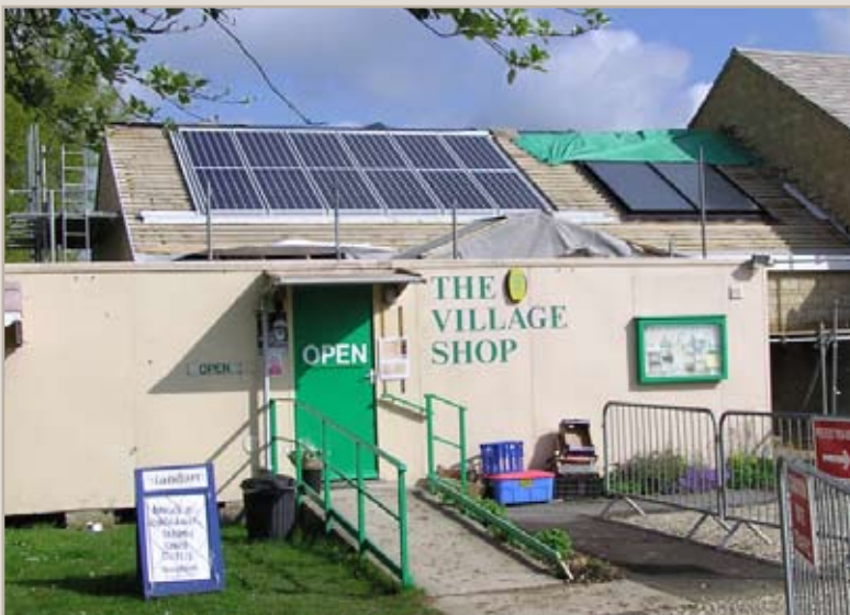
Solar panels being fitted to the new shop at Down Ampney, located just behind the portable building that's been used for the last 12 years.
